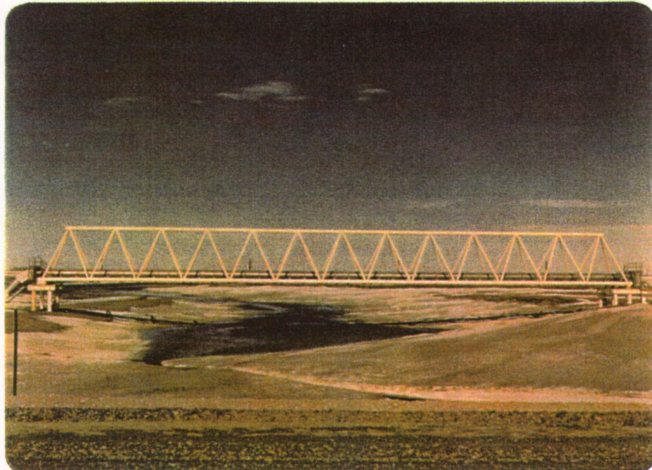
PHOTO 40 SINGLE-SPAN BRIDGE BP/SOHIO's crossing of the Putuligayuk River. Another crossing of the same stream further downstream uses regular mile-by-mile piles. 107-7-22
