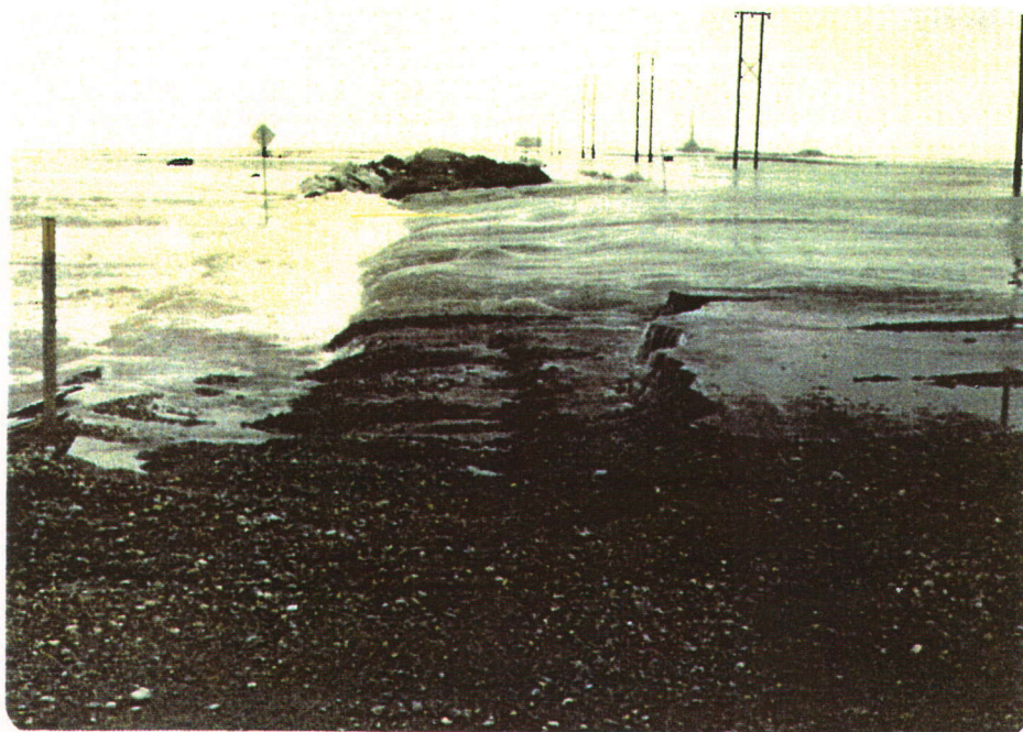
PHOTO 43 WEST CHANNEL SAGAVANIRKTOK RIVER Close-up of washout of gravel roadway sections shown above. 65-6-25
