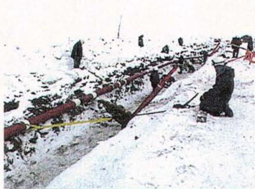
Reburial of TAPS Fuel Gas Line segment that had experienced upheaval buckling. (1998)
