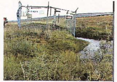
Thermokarsting ... adjacent to TAPS Fuel Gas Line Gate Valve 6. (1998)
