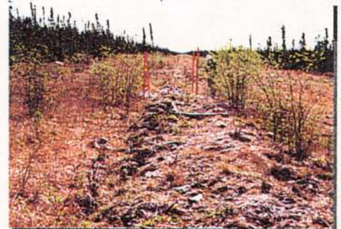
Coarse fill material placed over pipe to try to prevent further exposure and to protect pipeline ...Interprovincial Pipe Line System Norman Wells Right-of-Way.
