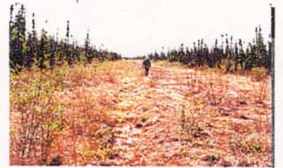
Heaving of backfill over pipeline ... Interprovincial Pipe Line System Norman Wells Right-of-Way.
