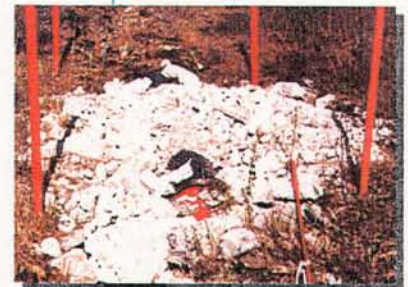
Section of exposed pipeline with half steel pipe section and rock over top for protection. ...Interprovincial Pipe Line System Norman Wells Right-of Way.
