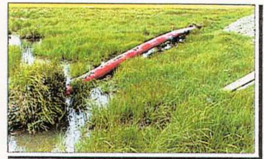
Upheaval buckling of the TAPS Fuel Gas Line. (1998)
