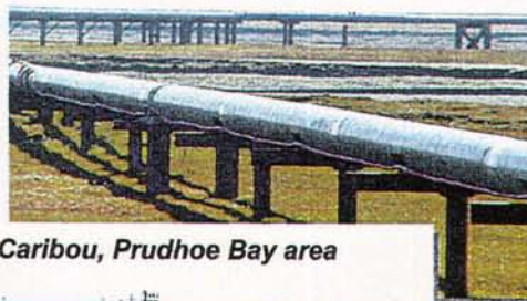
Eileen West End (EWE) Pipeline
