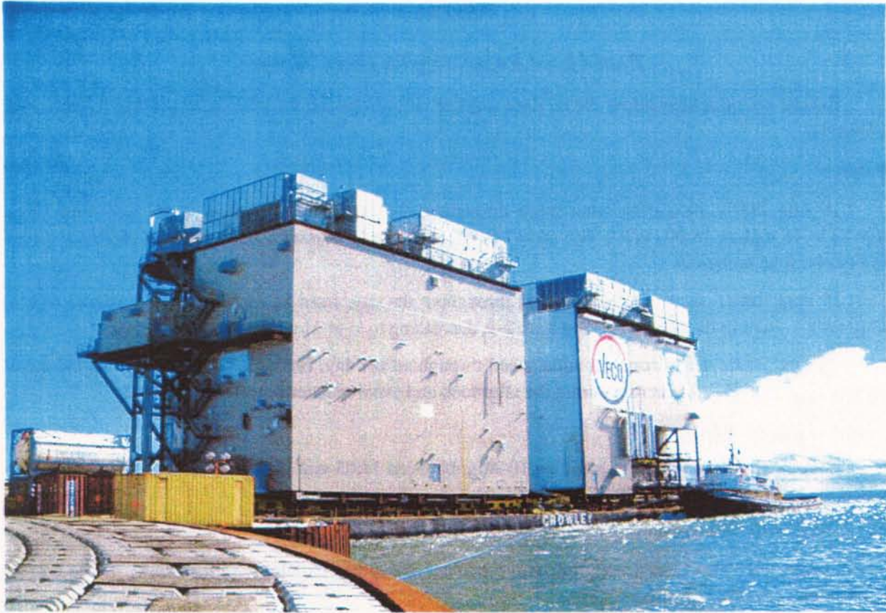
FIGURE 7.4. Sealift barge 400, with the N and S process modules, upon its arrival in Prudhoe Bay on 10 August 2001. The Ocean-class tug Navigator can be seen holding the barge on one side.
