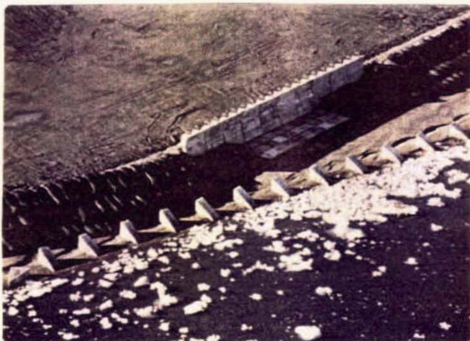
PHOTO 26. INNOVATIVE SLOPE PROTECTION SYSTEMS ON ALASKA ISLAND DRILLING PAD.
